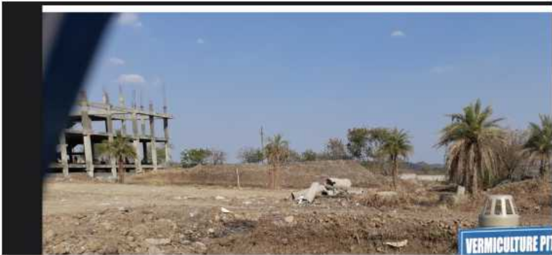
Sewage Treatment Plant
